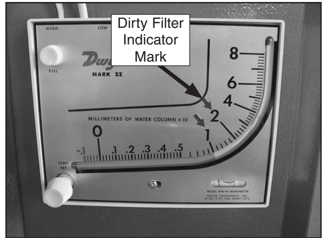
Figure 20. Dirty filter mark example.
